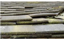
Bats will enter roofs through gaps in tiles
